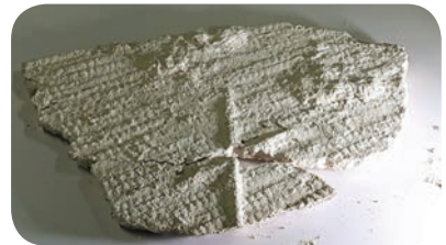
Piece of mortar taken from the collapsed transverse arch of the nave
